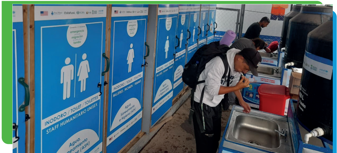
People in migratory transit make use of the sanitary facilities and have access to safe water (WASH component) of the Consortium LIFE-Honduras.
